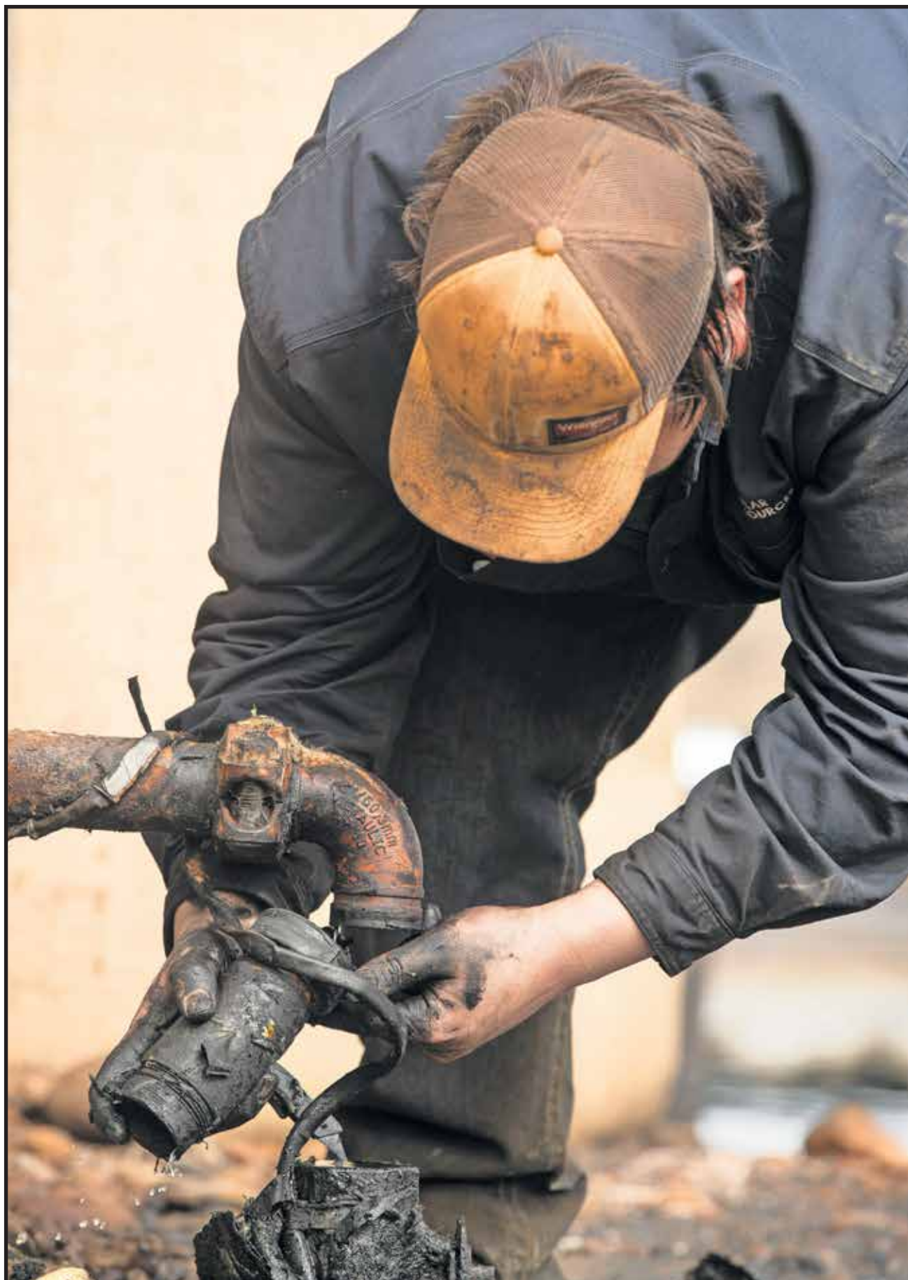
Jordan Moran works on fixing a broken pipe that connects to the injection pump housing containers.
