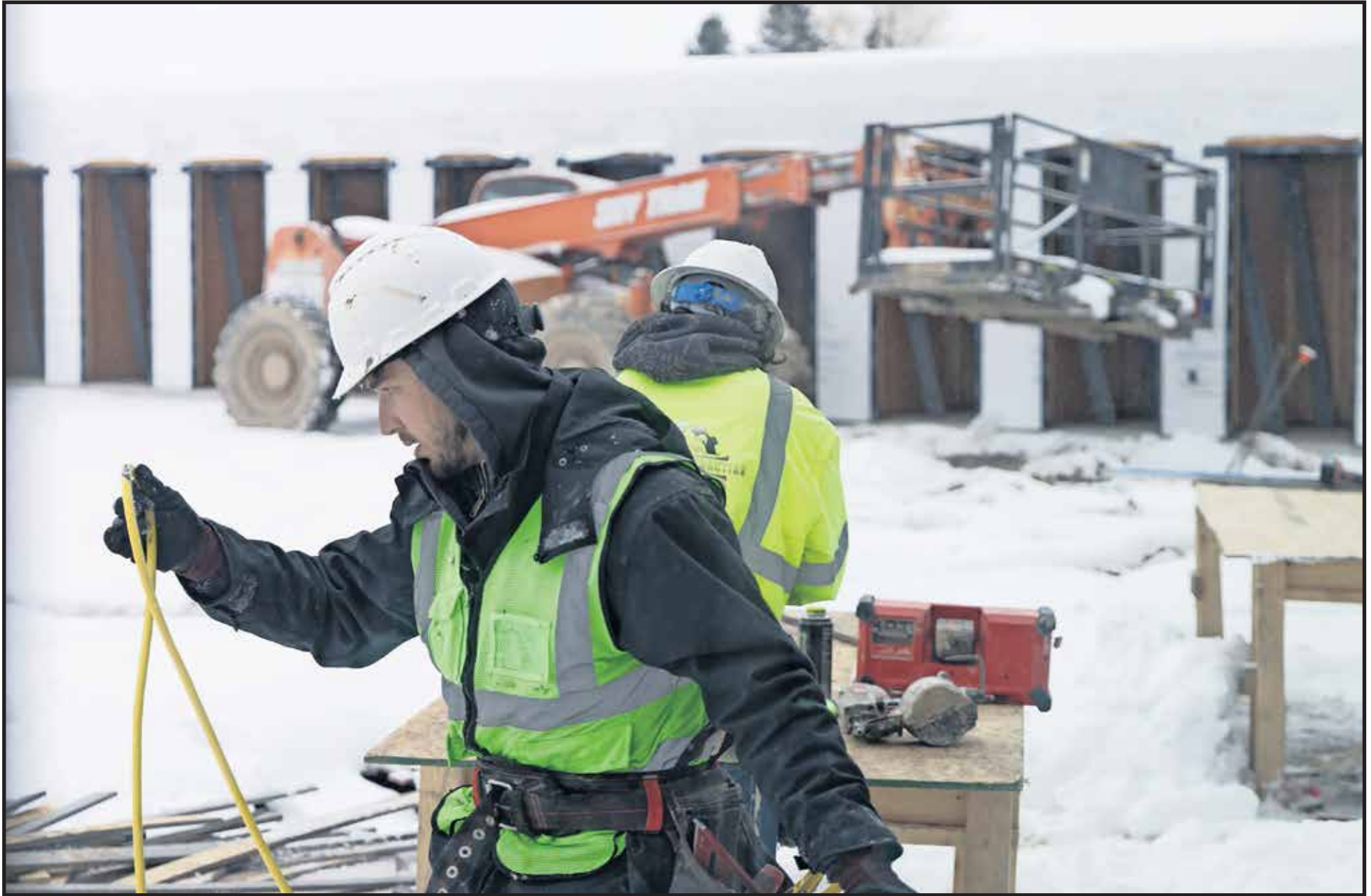
Two Sparrow Group employees help construct the additional storage units outside the reunification family housing facility in Pablo.
